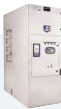
Retrofit, 4.16KV, 8BK20 exsiting bus-bars, 1600mm (63") Depth
