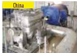
China Liquid Gas Booster Compressor 6600V / 600A
